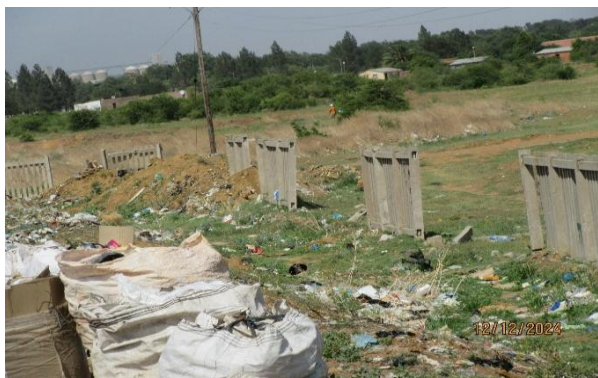
Figure 3.1: Precast concrete panel fencing vandalised in the Viljoenskroon landfill site
