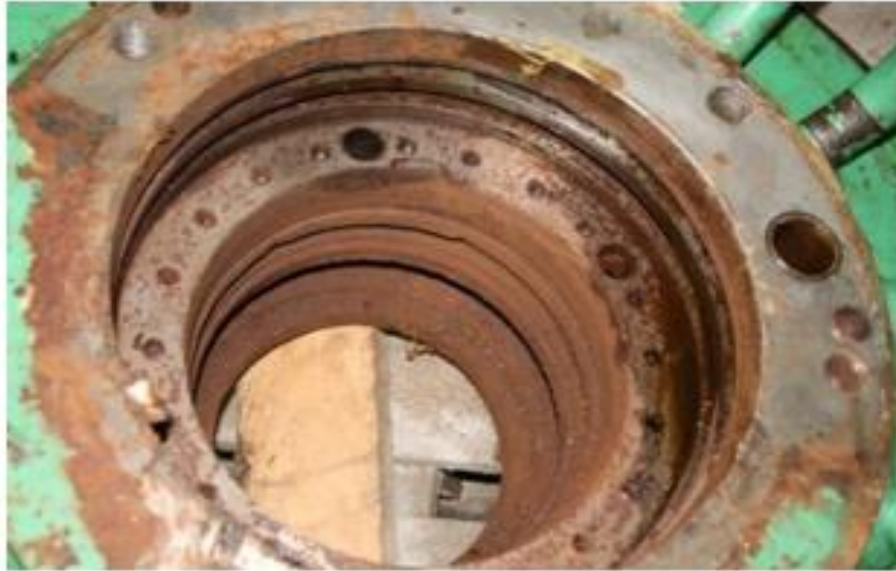
Figure 6: Corrosion of the cover seal location
