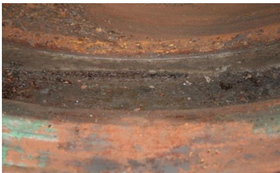
Figure 5: Corrosion of the shear ring groove
