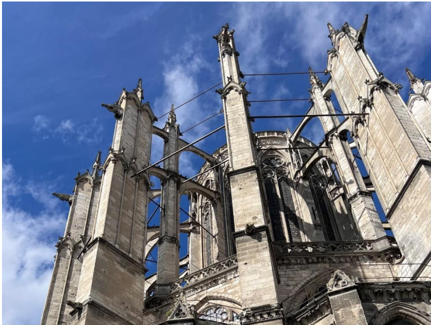
Figure 4. Flying Buttresses and Iron Tie Bars Added to Reinforce the Structure After the Collapse of the Choir in 1284 (Photograph by the Author).
