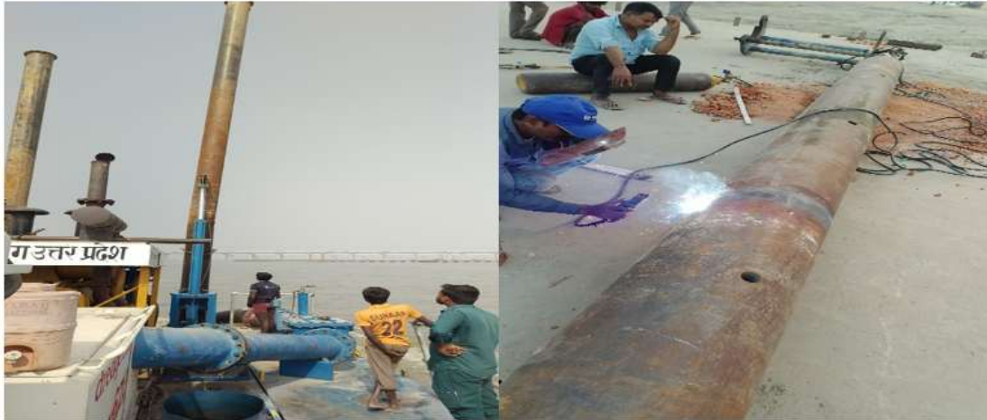
Figure 20: Bending of Dredger Spud
