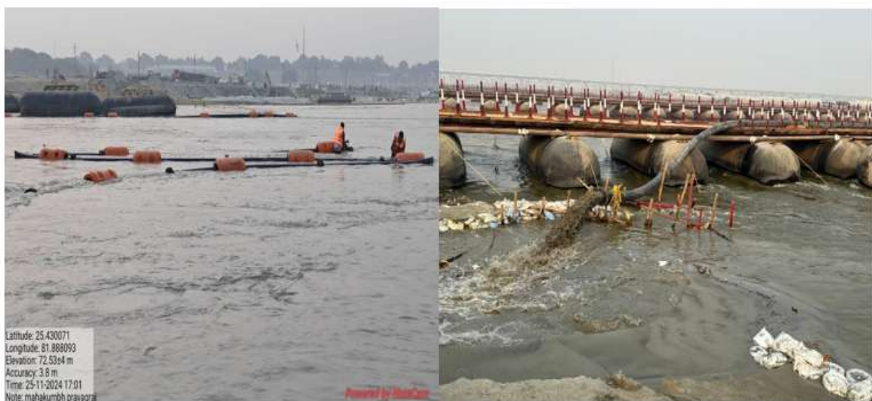
Figure 19: Bending and Breaking of Discharge Pipes
