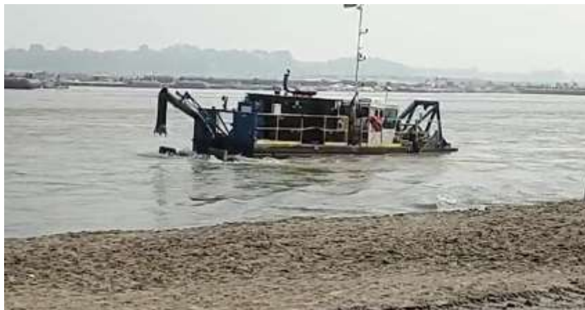
Figure 14: Dredger IMS 8012 Unstable due to High Velocity Discharge in Channel
